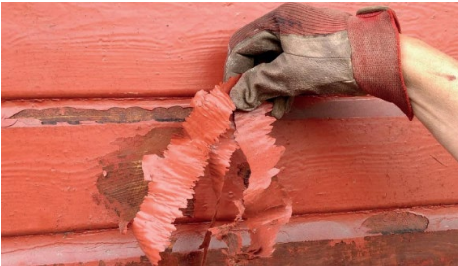
Figure 3. Layers of red plastic paint peeling off in larger flakes.
