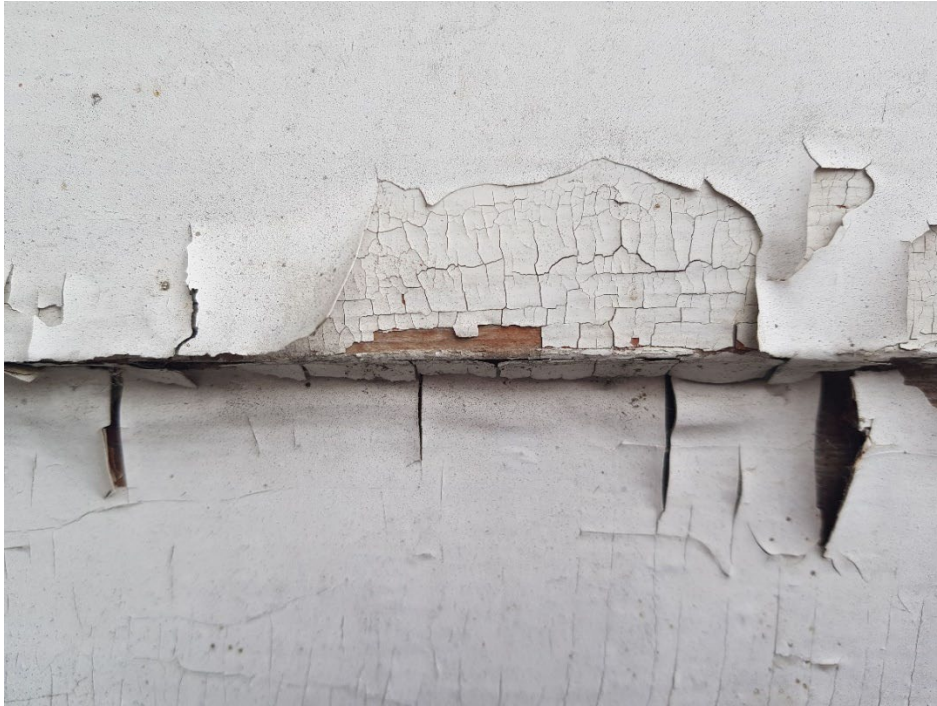
Figure 4. Modern paint cracks in larger flakes. The underlying linseed oil paint develops a crazed pattern, almost resembling alligator skin.
