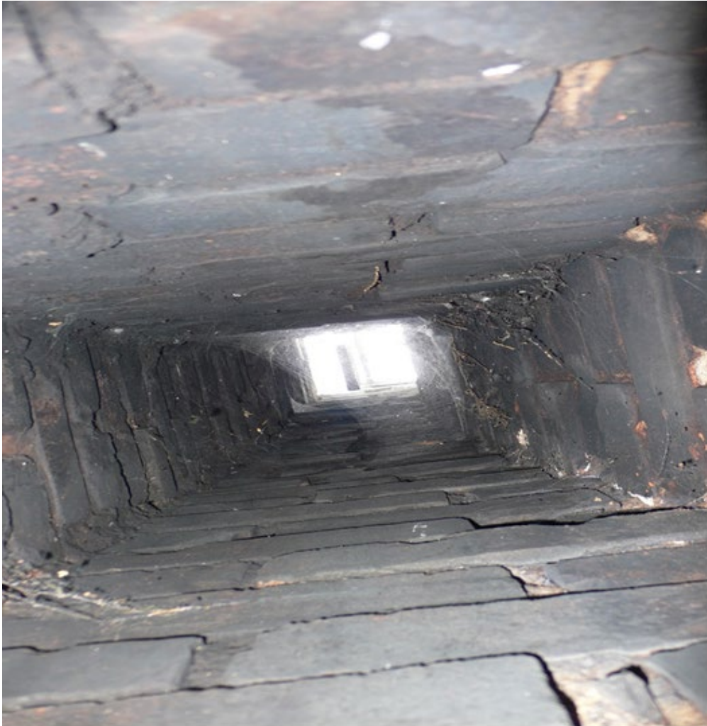
Figure 23. The image shows a soot flue, which is an example of a chimney where a cap may be necessary to protect against moisture damage. By preventing moisture penetration, you can extend the life of the chimney and avoid costly repairs.
