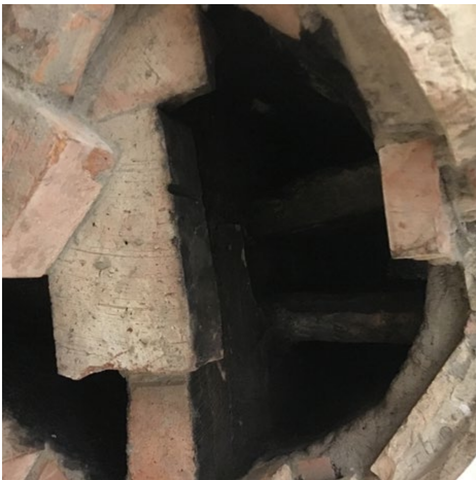
Figure 9. This is what a normally sooty flue looks like.
