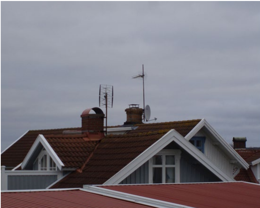
Figure 35. Two houses from the same period, but with different solutions for chimney repairs.
