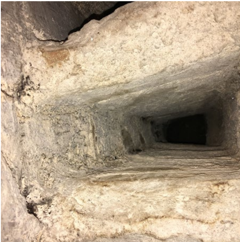
Figure 11. This is how it should look the day after the NHL 5 mortar has cured and become much whiter than the day before, with most of the soot gone.
