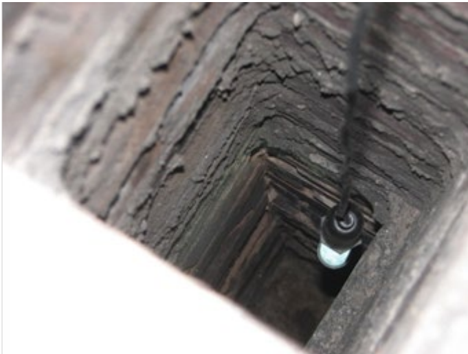
Figure 8. Here you can see how to illuminate the sides and see how the joints have loosened.
