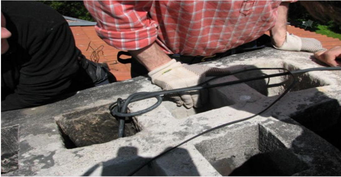
Figure 1. Picture of chimney flues 12x12 cm.
