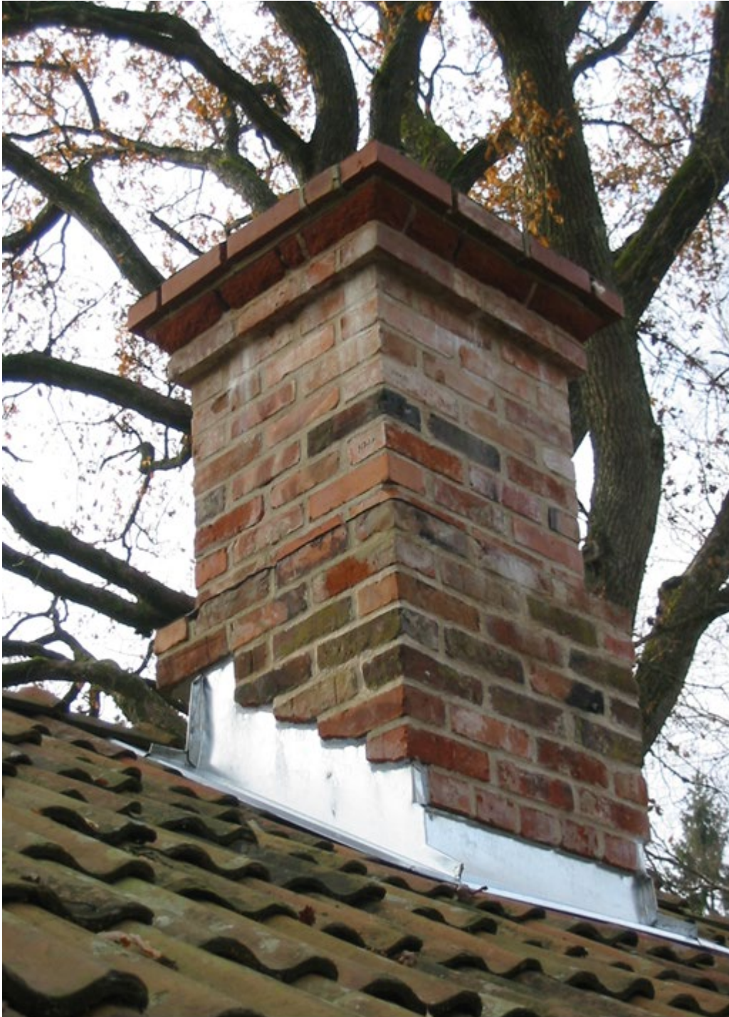
Figure 25. The image shows a rebuild where the old bricks have been reused to rebuild the crown. At the base of the chimney, plaster has been chosen, creating a smaller overhang, and the overhang has then been fitted with a metal flashing for protection. The biggest deviation from the original is that legislation now requires a higher chimney, which has led to two extra courses of bricks being added on top. These new bricks have a different colour and firing, which differs from the reused bricks. Additionally, these new bricks have been mortared with a mortar that weathers over time.
