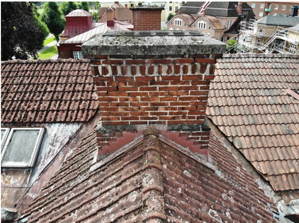
Figure 33 and 34. The images show a house from 1899 where the chimney has been repaired. Unfortunately, the rebuilding of the crown was done without documenting the type of stone, and thus the original tilt and the house's typical "king's crown" design were not preserved. Despite making an overhang to retain
