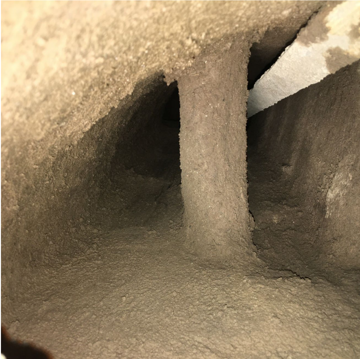
Figure 16. The right flue is perfect; you can see the contours of the bricks. The joints are well-filled. The left one is acceptable with occasional bulges.
